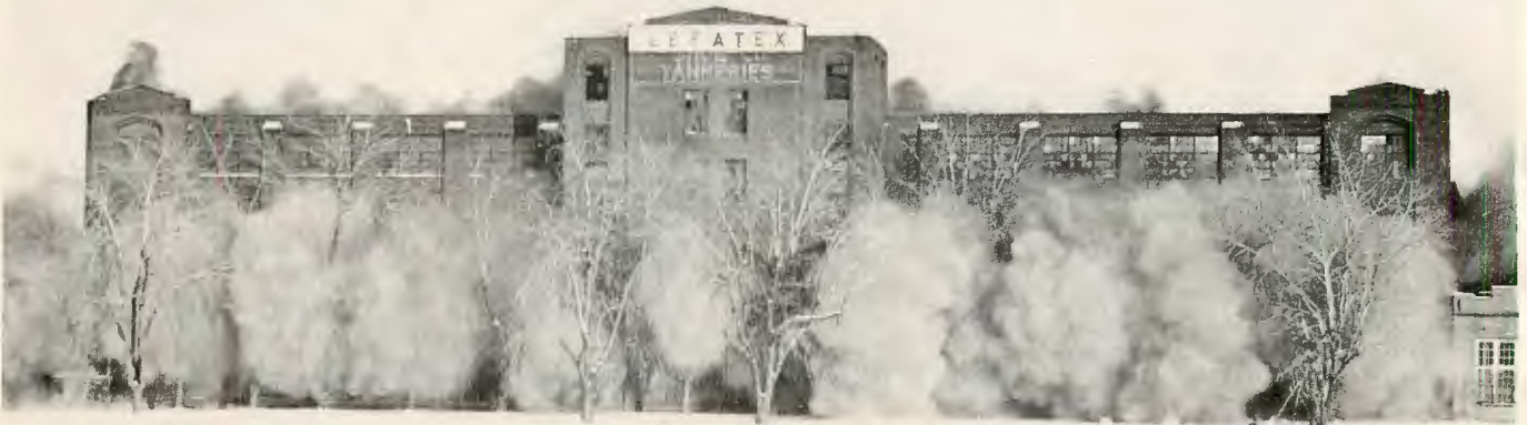
Initial blast. Charge detonated from outside to center. 127 pounds of gelatin dynamite were placed in 257 locations.
